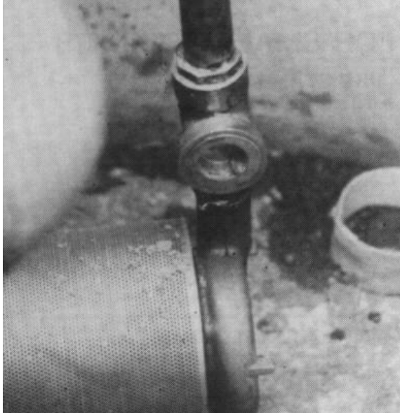
Algarid on a submersible pump in a water channel sump
